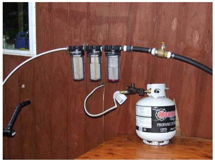
Filters hung up above the propane tank for the range
